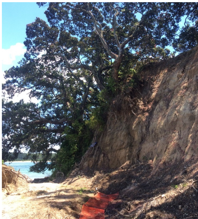
Photo 6. The slip site. Showing large pohutukawa.
